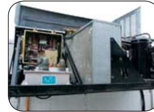
Installs next to condenser
